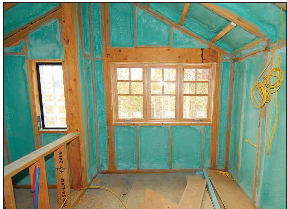
Interior view of Breckenridge's first custom net zero home using Boise engineered lumber which allowed for wider stud spacing and 30 percent more sprayed foam insulation in exterior walls and ceilings.
