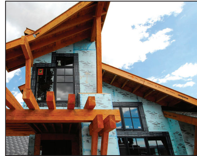
This 8,000 sq.ft. Breckenridge luxury home is designed be one of the most energy efficient residences in Summit County.
